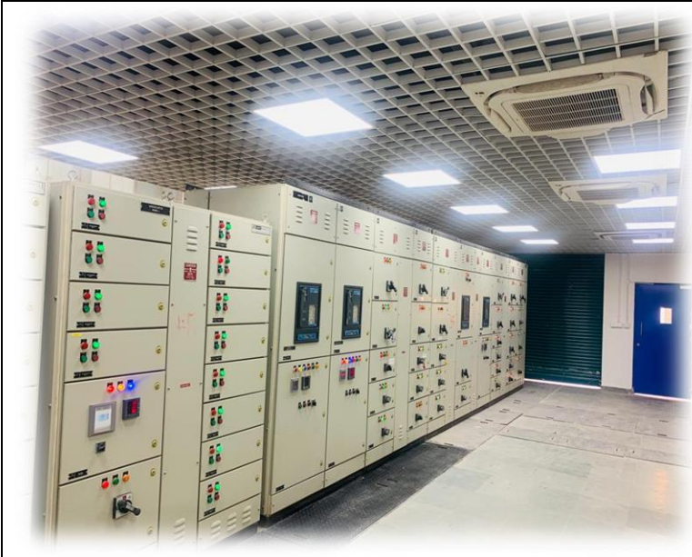
LT Panel Room - M/s. Mastek Ltd. - Mahape - Navi Mumbai.
