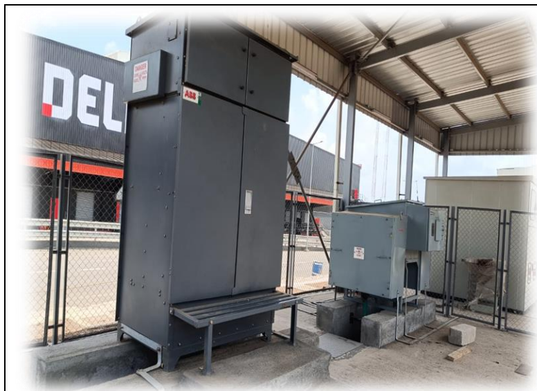
HT Sub Station Works - Welspun One Logistics Parks Pvt. Ltd. - Bhiwnadi
