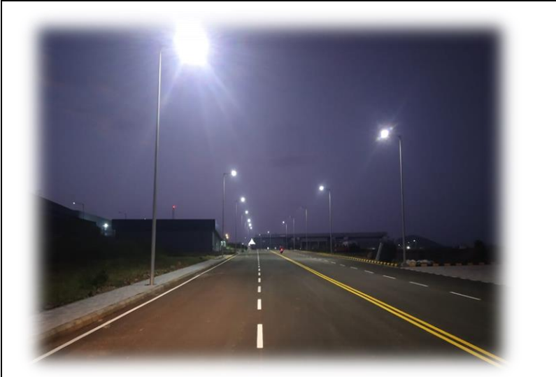
External Lighting - Indospace - Chakan - Pune
