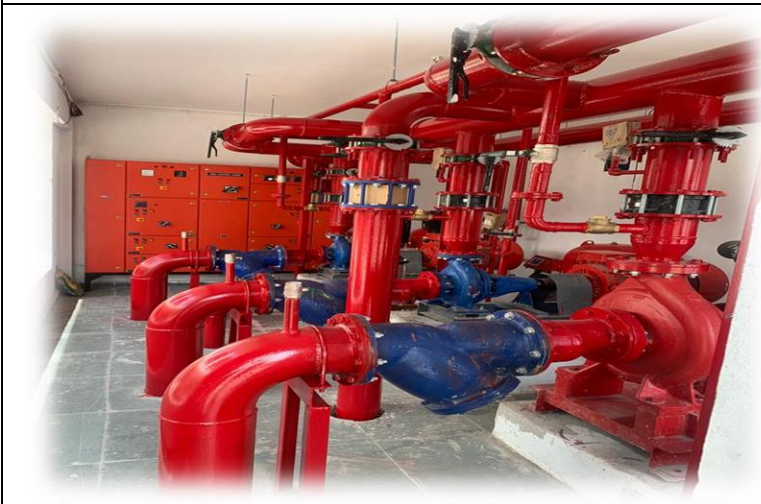
Fire Fighting System - M/s. Mastek Ltd - Mahape - Navi Mumbai
