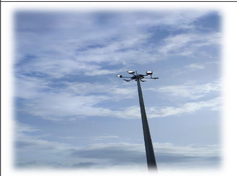
High Mast Poles - Indospace - Chakan - Pune
